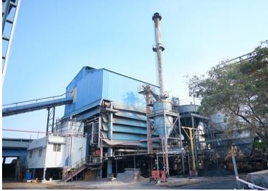
16 TPH Solid Fuel Boiler
